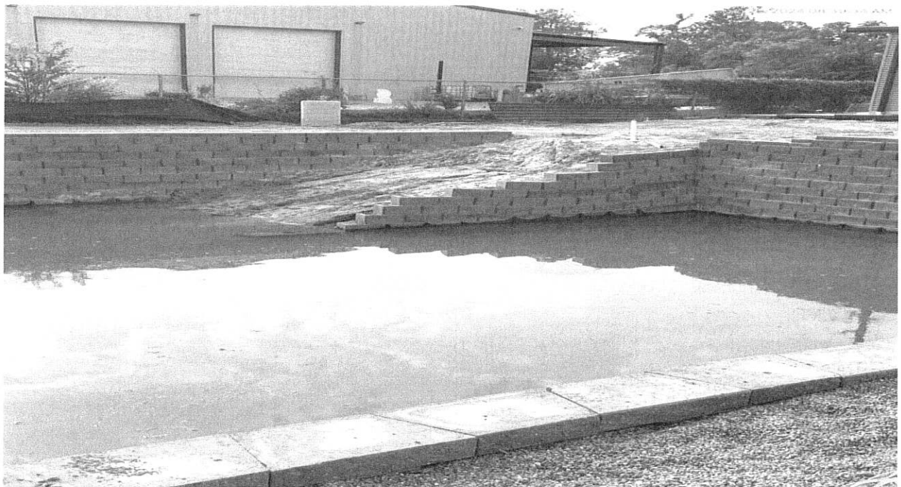
8/22/24 Detention pond ramp wall issue
